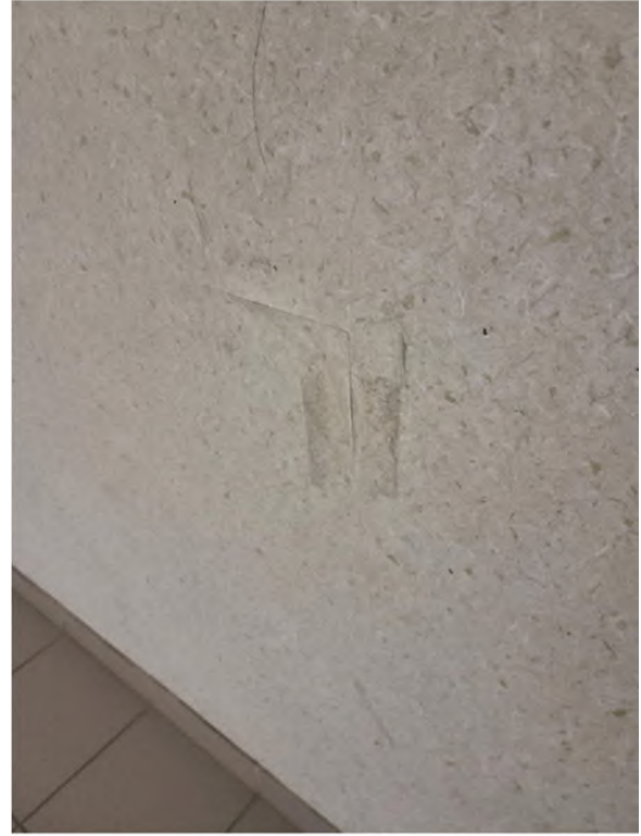
Photo 67 Minor cut on the wall
