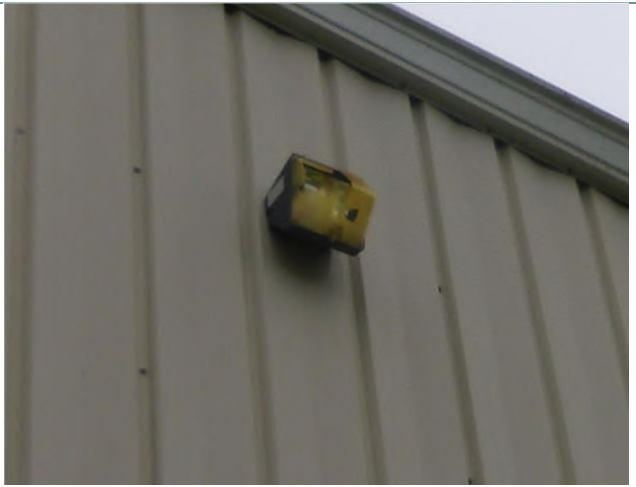
Photo 68 A light fixture at the back of the building has a broken lens and possibly broken lamp
