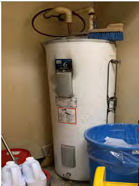
Photo 29 Lobby/Kitchen hot water tank
