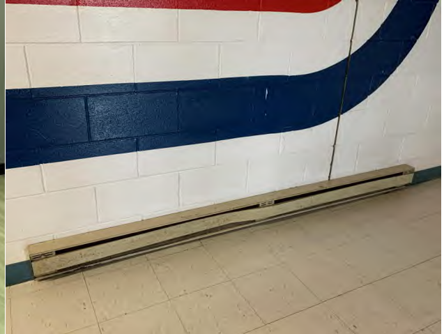
Photo 52 | Old electric baseboard heaters
