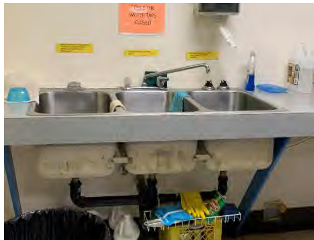
Photo 30 Kitchen plumbing fixtures
