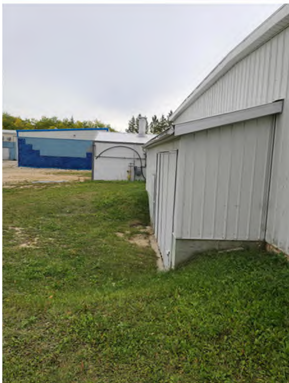
Photo 45 A damaged gutter
