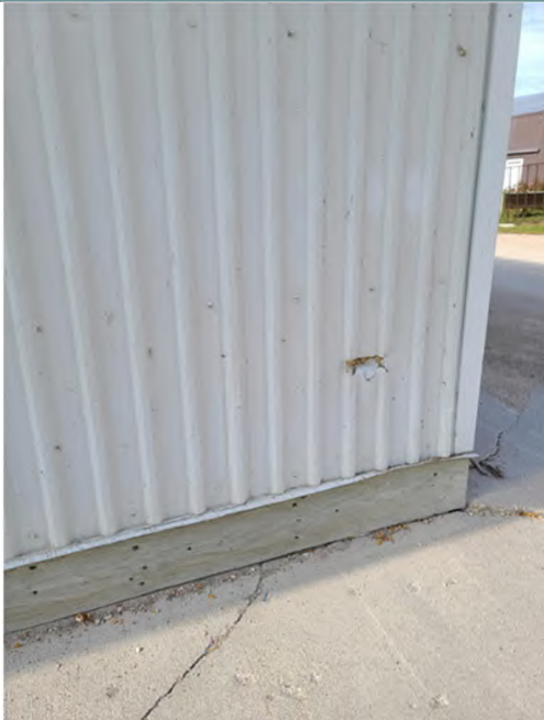
Photo 110 Damage to insulated panel
