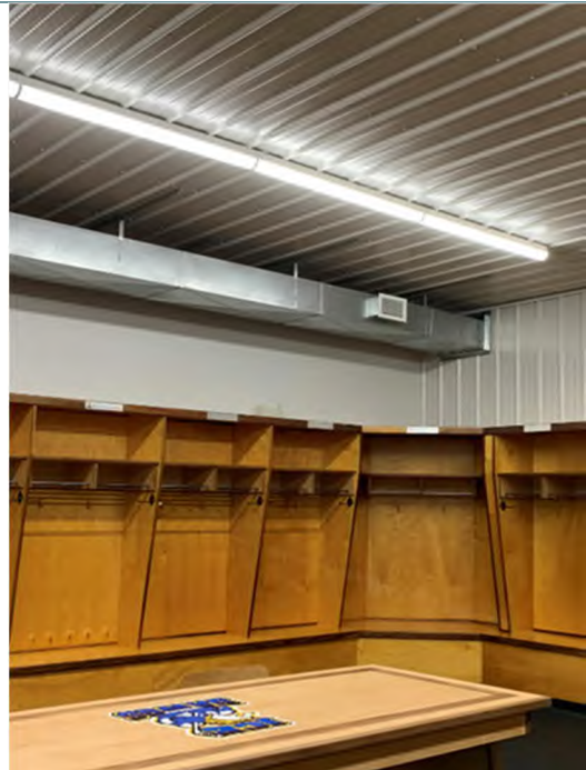
Photo 18 Dressing room duct work and grilles
