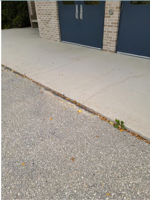
Photo 64 A small step between concrete apron and asphalt
