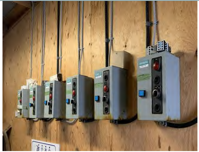
Photo 38 Aquatic Centre panelboards
