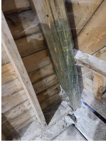
Photo 111 Gaps underside of the exterior wall allowing air flowing into the building
