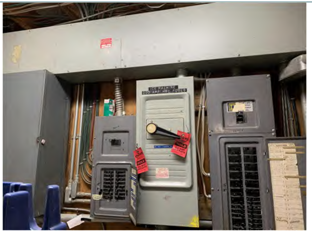
Photo 48 | Curling Rink panelboards
