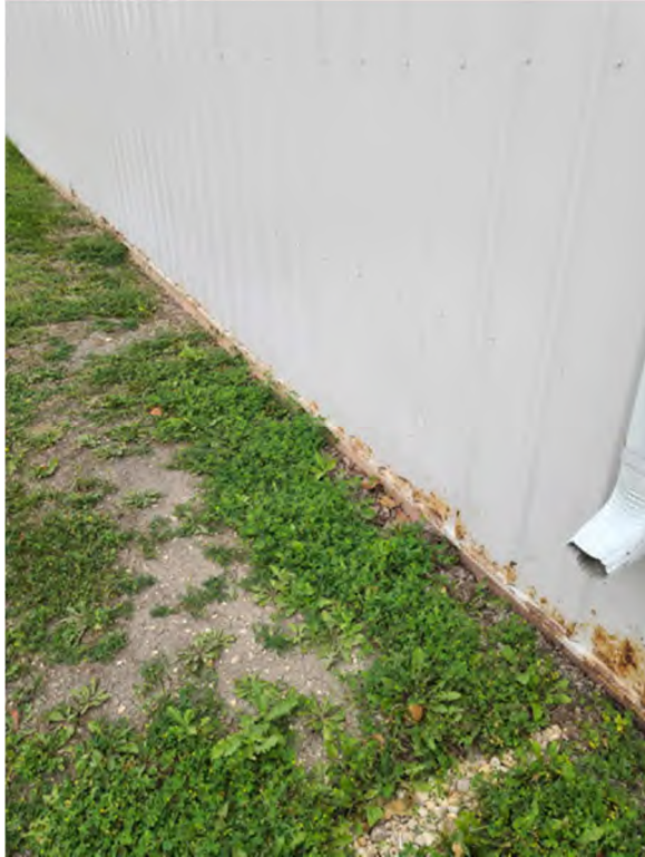
Photo 43 Rust observed at the base of the exterior wall panels
