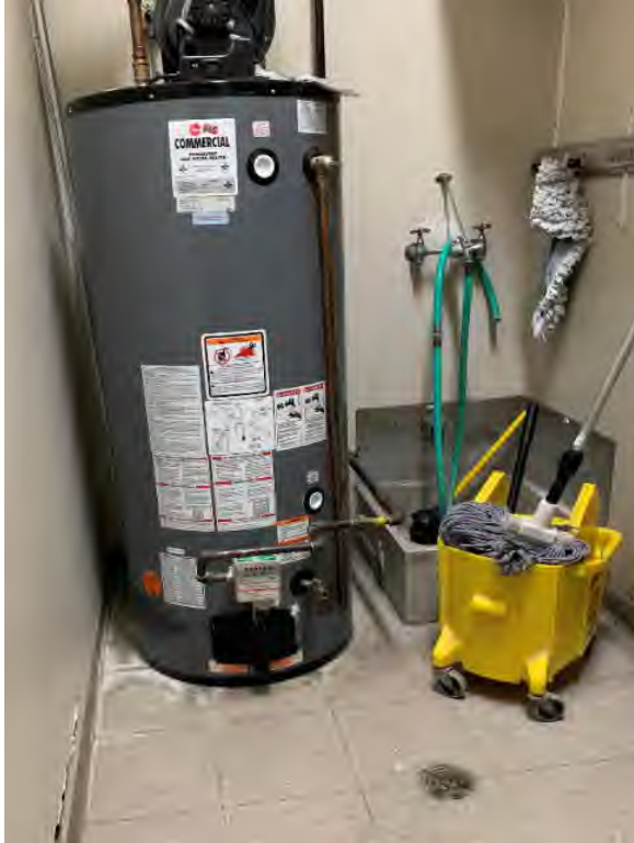
Photo 75 Hot water tank
