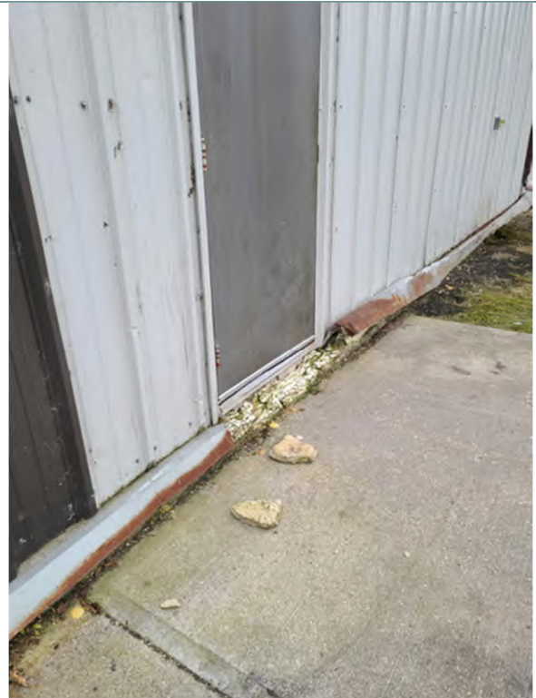
Photo 81 Heaving of board insulation pushing up flashing at the base of the walls
