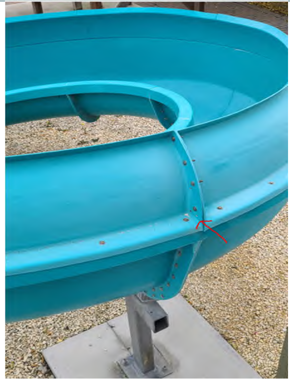
Photo 40 Two bolts are missing at one of the connections of the slider
