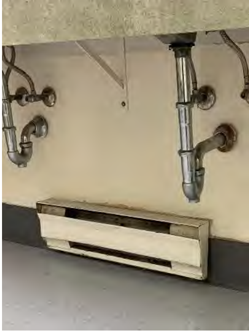
Photo 16 Bathroom baseboard heater
