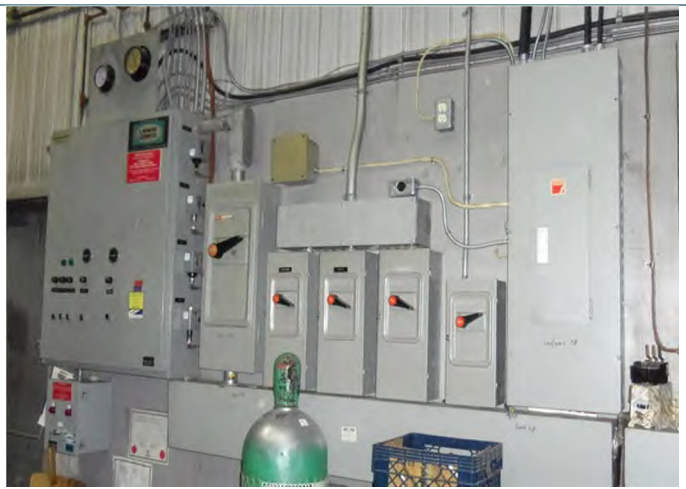
Photo 8 | Ice plant electrical distributor
