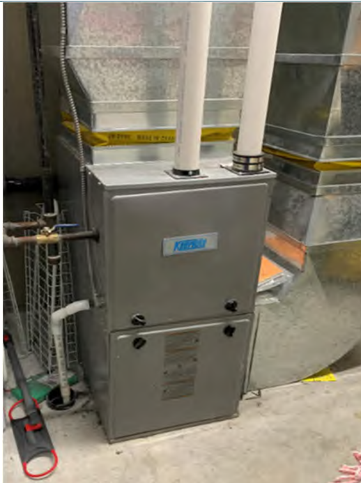
Photo 17 Dressing room furnace
