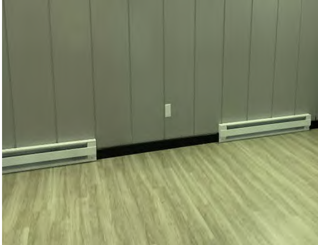
Photo 51 | New electric baseboard heaters
