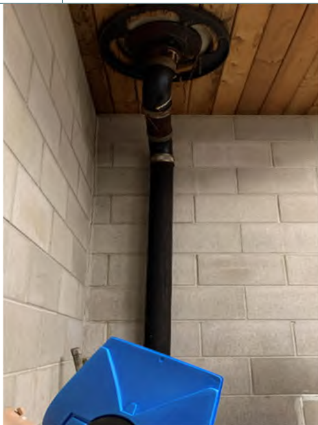
Photo 61 | Mechanical room storm pipe
