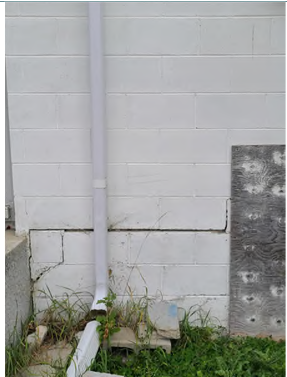
Photo 42 | Cracks in masonry joints
