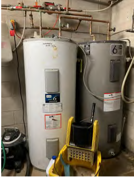
Photo 27 Field house hot water tank
