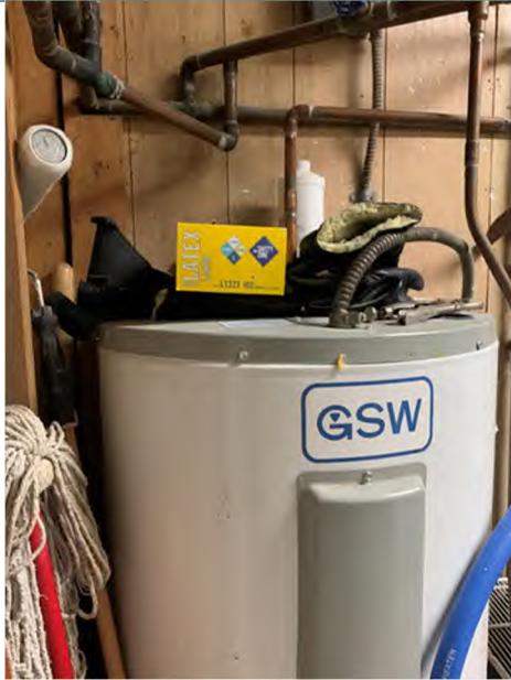
Photo 59 | Curling Rink hot water tank
