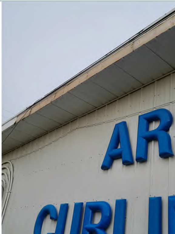
Photo 41 | Missing fascia cover at the Curling Rink
