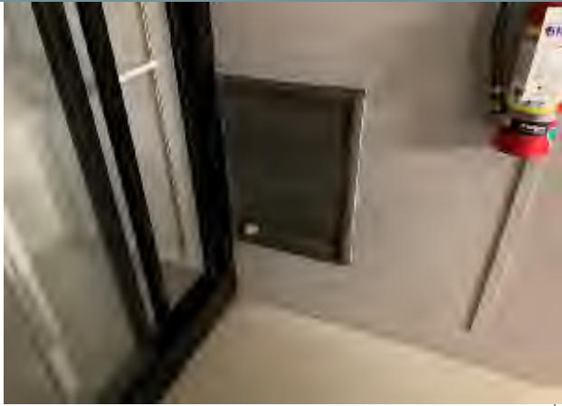
Photo 53 | Curling Rink entrance electric heater
