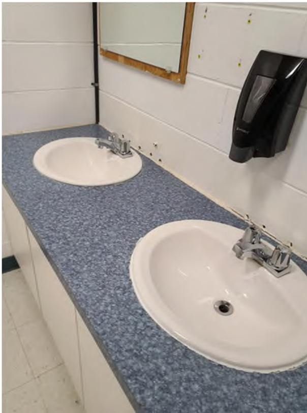
Photo 46 Holes on walls in men washroom
