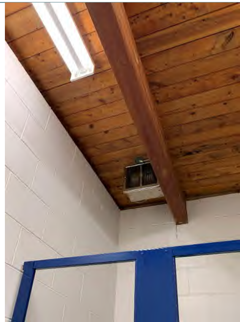
Photo 50 | Curling Rink washroom fan
