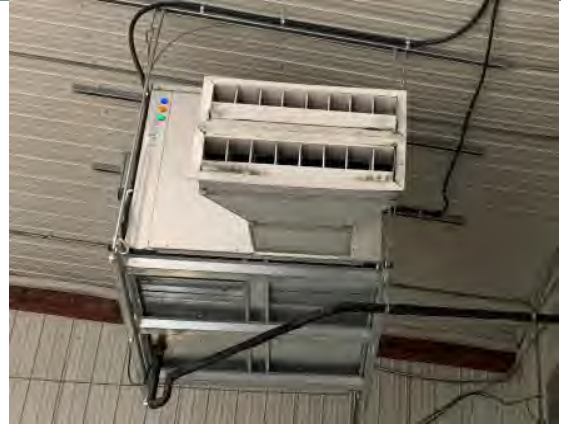
Photo 20 Ice Rink intake damper
