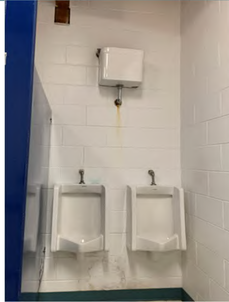
Photo 60 | Main washroom plumbing fixtures
