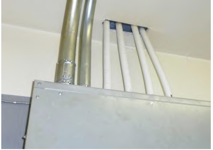
Photo 7 | Cable and conduit transit – Electrical Room # 3
